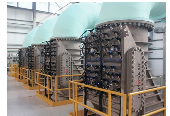
Figure 21. UV drinking water plant.
